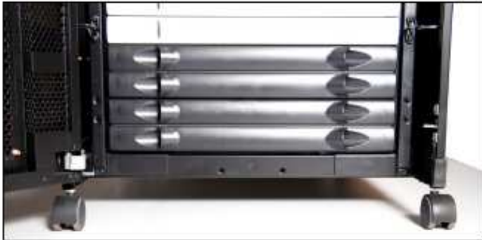
Rack With No Seal Air can freely flow under rack
