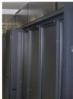
Removable panels for future rack expansion.
